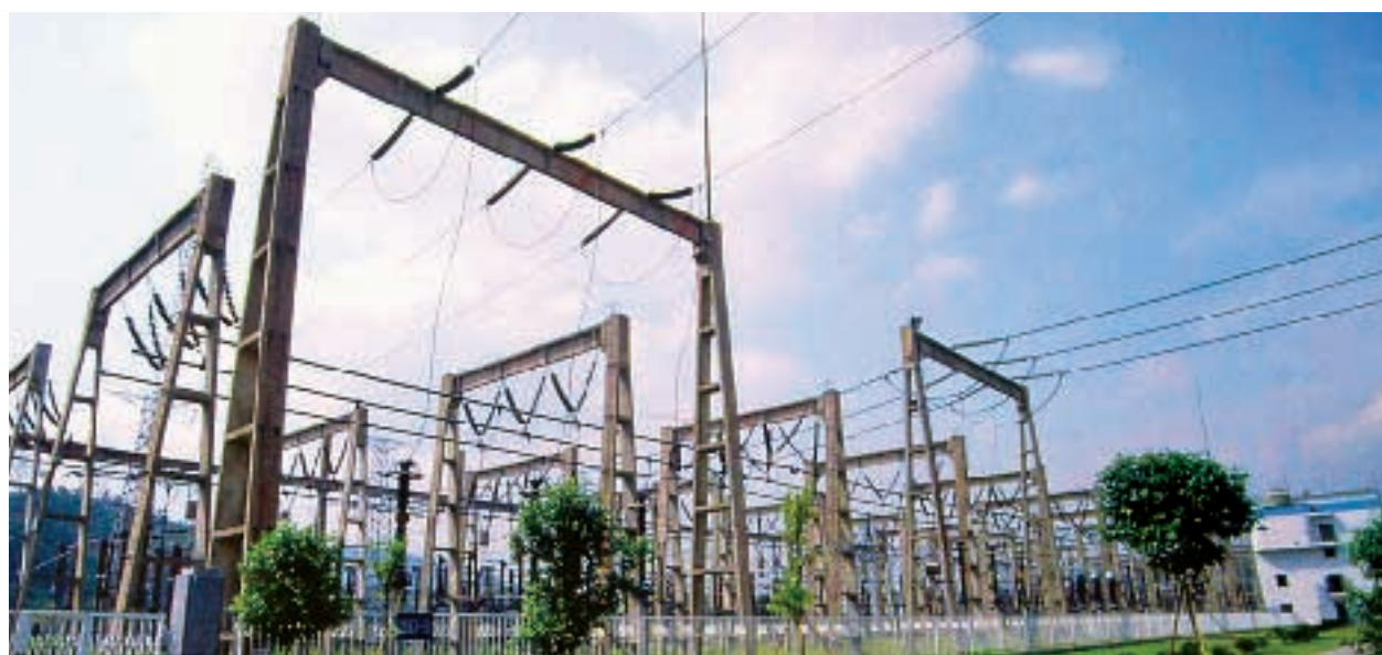
Zhujiang Power Station
