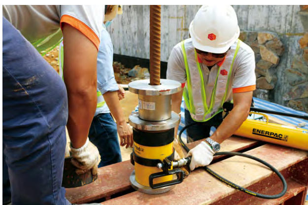
The Laboratory and Testing Department of New World Construction Company Limited carries out a proof load test
