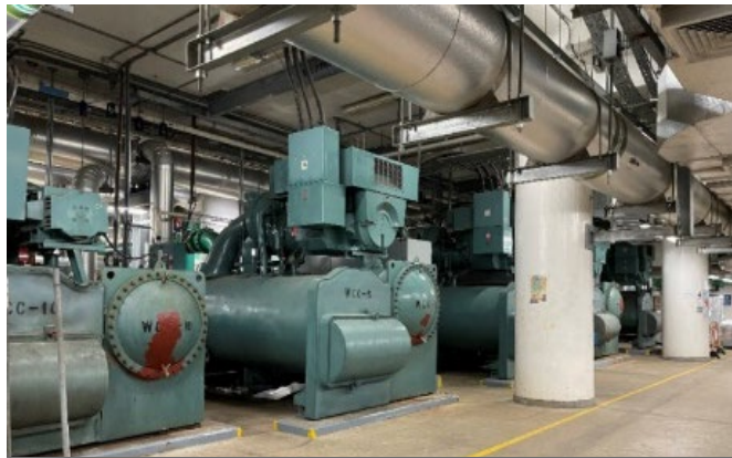
Smart Building Management System, e.g. Chiller
