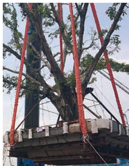
Tree conservation through transplanting at a Public Housing Project in Queen’s Hill, Fanling
