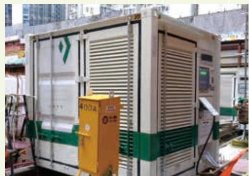
Use of "Enertainer" at construction sites
