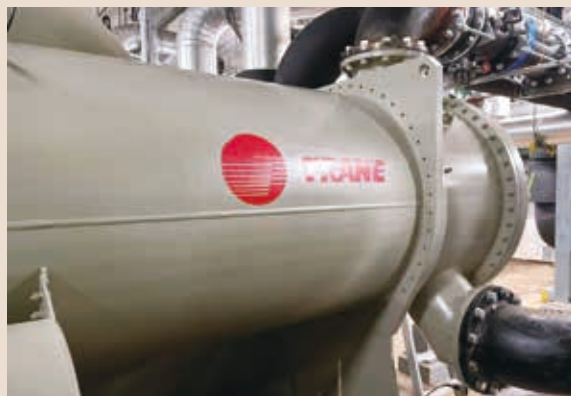
Two 2500TR chillers replaced in FY2022
